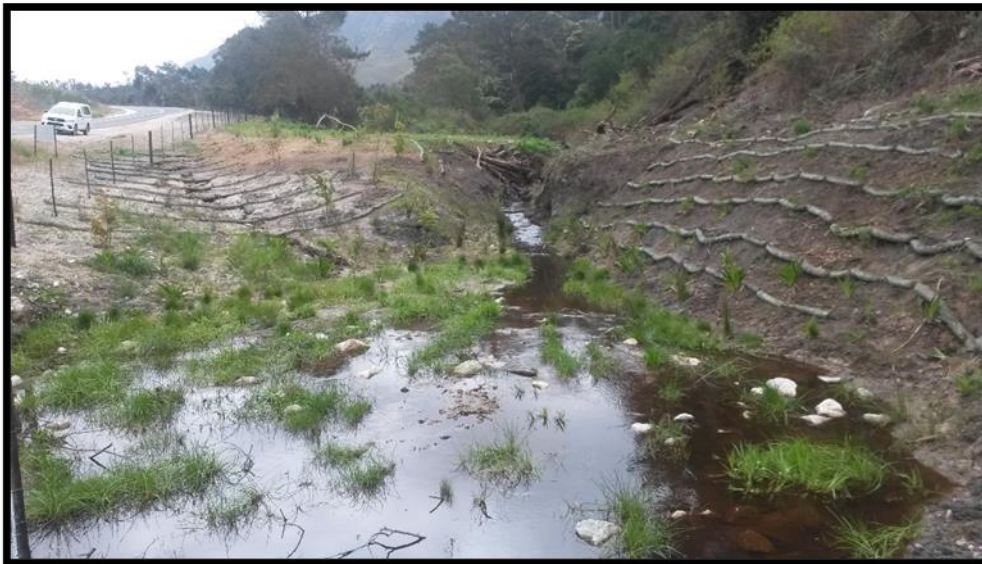
Figure 10: Example of horizontal terracing with biodegradable sausages to reduce down slope erosion.
