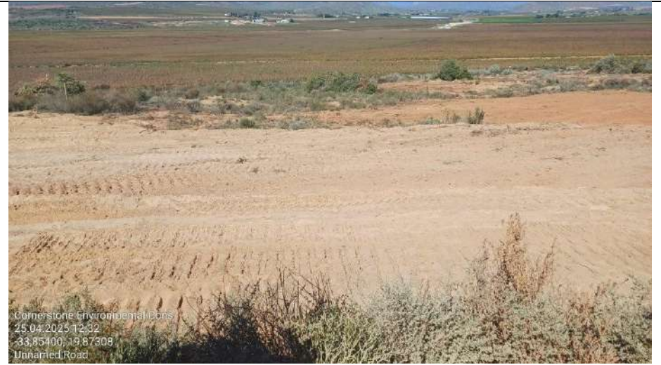
Photo 4: Looking south over the recently cleared section of Area 2 that falls within the aquatic buffer. This 4800 m 2 area was wrongfully cleared and will be rehabilitated.
