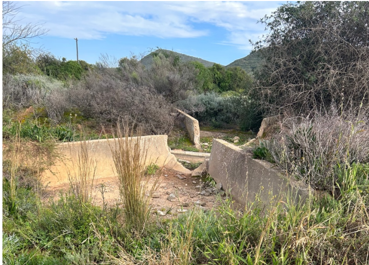
FIGURE 2: LE CHASSEUR & GOREE CANAL RUNOFF BRIDGE - DAMMAGED
