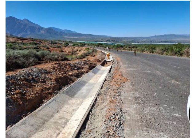
Road has now been tarred and stormwater drains are being completed. Minimal disturbance outside the site area was noted.
