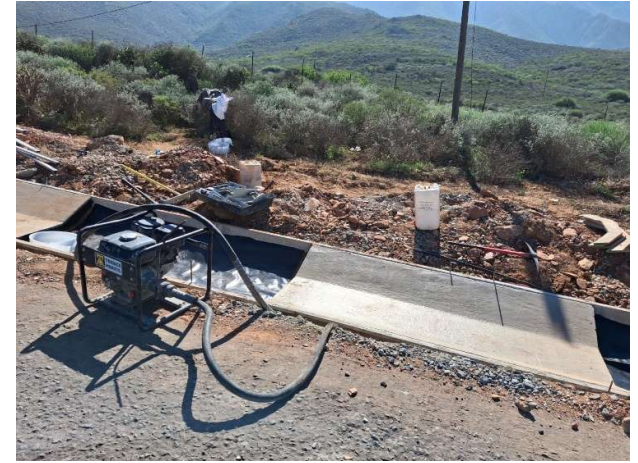
No drip tray beneath the generator.
