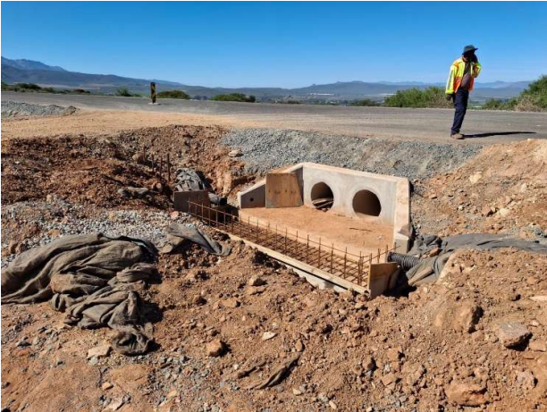
Culvert beneath the road. Loose shade netting must be removed from site or secured.
