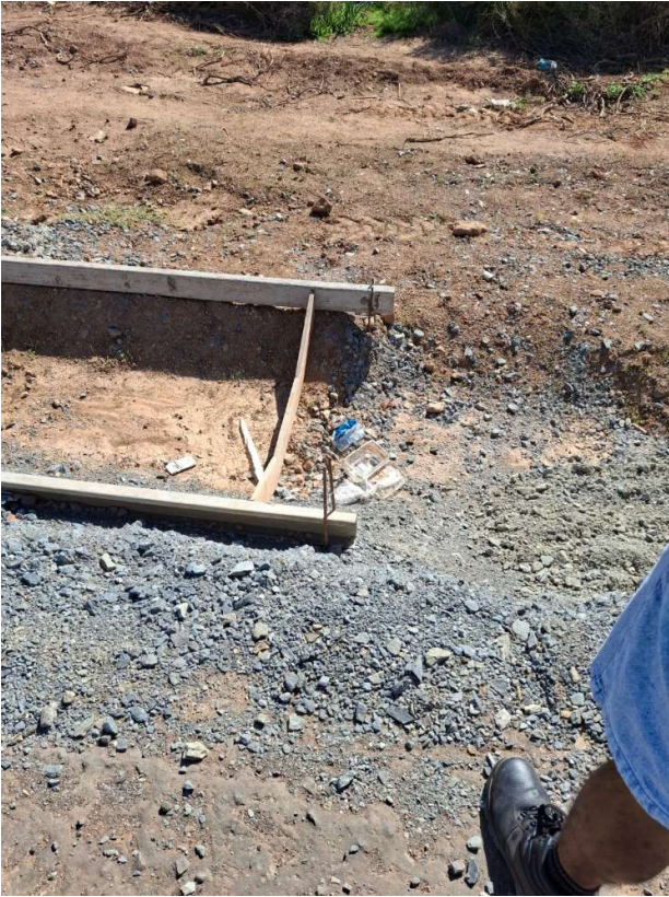
More litter noted on site.
