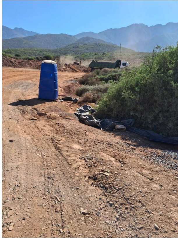
Mobile toilet at laydown area. Toilet needs to be secured to the ground. Loose plastic must be removed or secured.
