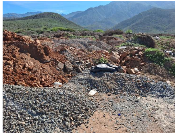
Stockpiles of material that will likely be disposed at a landfill site. Note litter. The nearby watercourse must be clearly demarcated to ensure stockpiles do not encroach within 32m of the watercourse.
