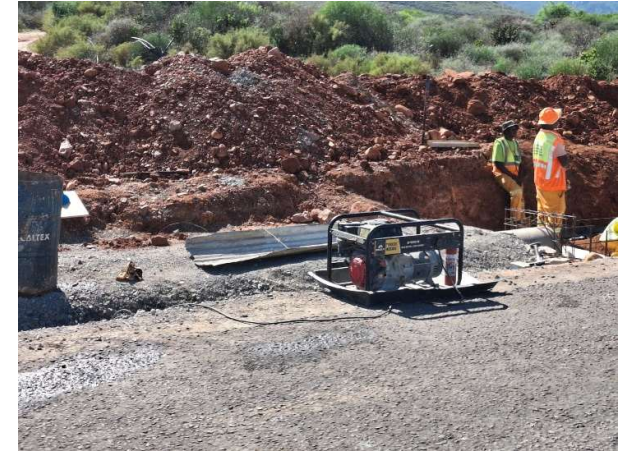
Drip tray in place.
