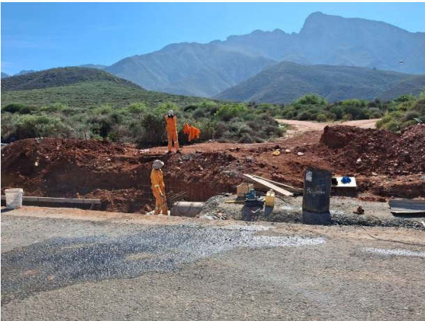
Drum provided for waste but surrounding area contains much litter.
